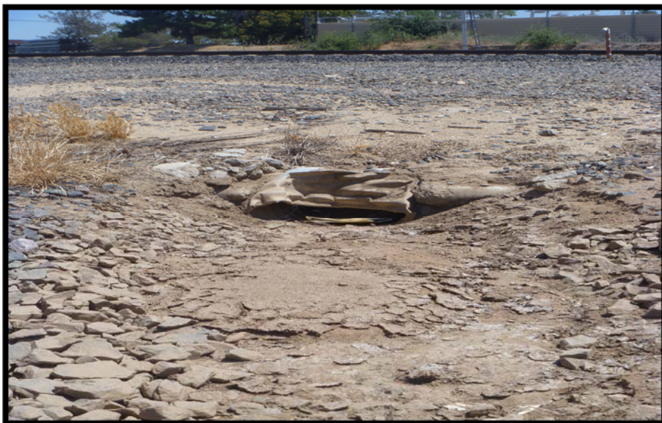
Photo 2 – Structural Ranking of 1
