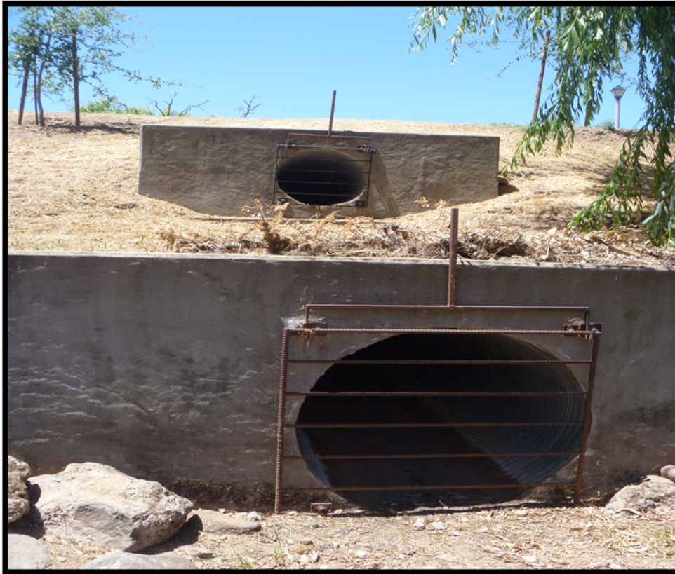
Photo 1 – Structural Ranking of 5
